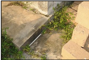
...emerging at the side of the porch in this conduit...
